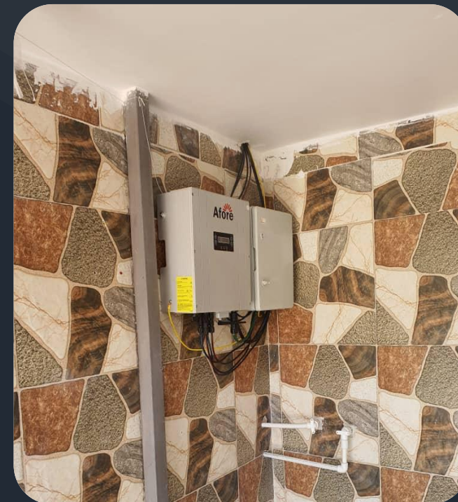
Country : Iran Product : Single-phase 5kW Project Size : 200kW residential community project
