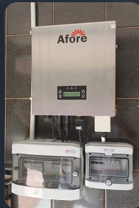
Country: Pakistan Product: Three-phase 6kW Project Size: 6kW
