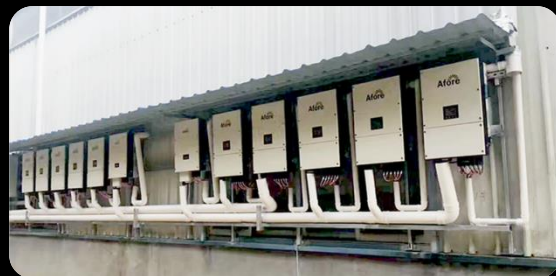
Product: Three-phase 20kW Project Size: 200kW
