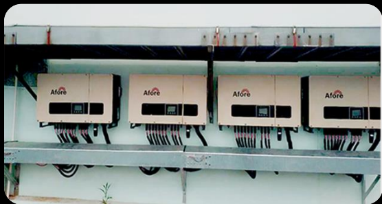
Product: Three-phase 60kW Project Size: 500kW
