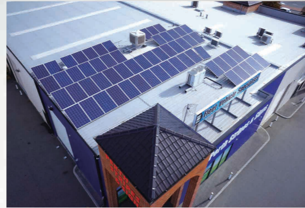
15kw Perth, Australia
