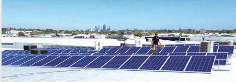
15kw Perth, Australia
